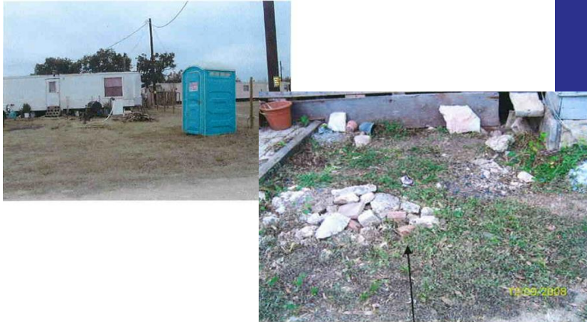
Septic tank lid under rocks
